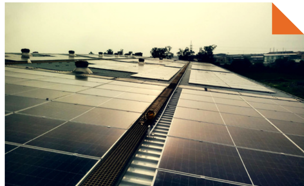
Embee Screens 378.36 kWp
