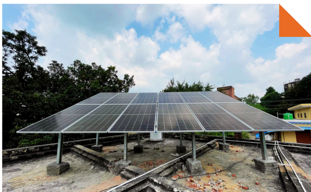
UPNEDA - Grid Tied Solar Plant 1400 kWp
