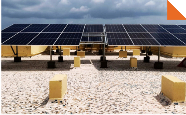
Shri Kolhapur Bhavan 49.5 kWp
