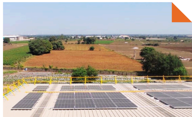
Max Power Engineers 49.5 kWp
