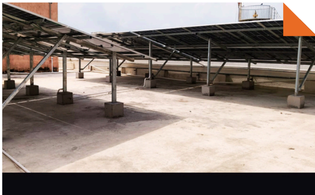
Shree Samdadi Bhavan 99.55 kWp
