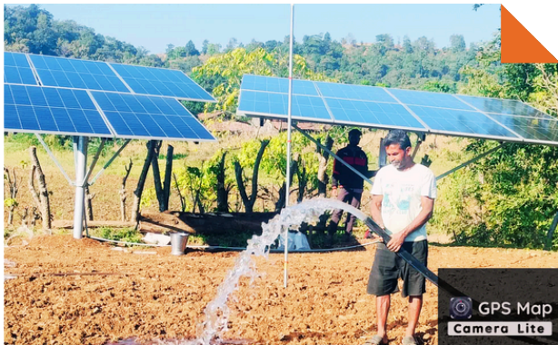
DGVCL 2760 nos Solar Water Pump
