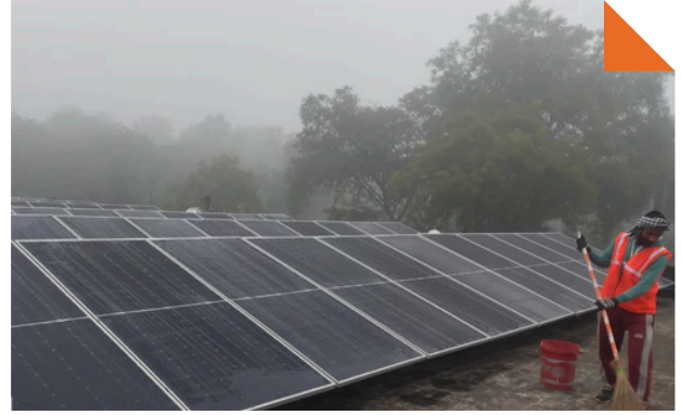
Rajasthan Electronics & Instruments Ltd. 700 kWp
