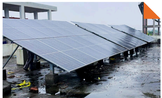
PEDA - Grid Tied Solar Plant 1470 kWp
