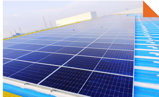
Ratnatris Pharmaceuticals (500 kWp)
