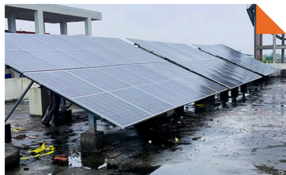
PEDA - Grid Tied Solar Plant (1470 kWp)
