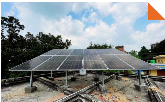
UPNEDA - Grid Tied Solar Plant (1400 kWp)
