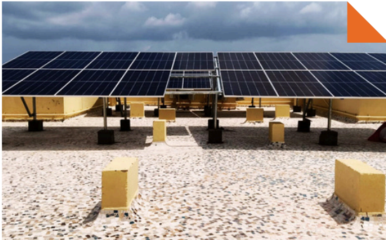
Shri Kolhapur Bhavan (49.5 kWp)
