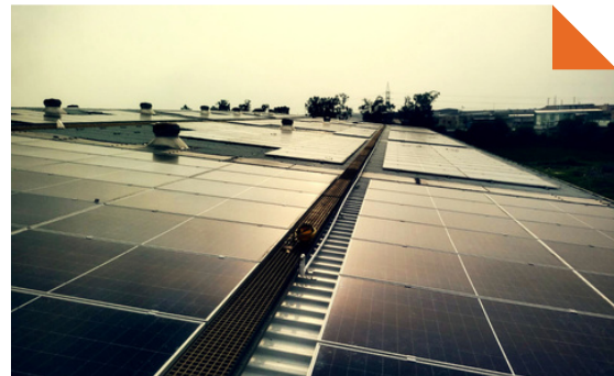
Embee Screens (378.36 kWp)
