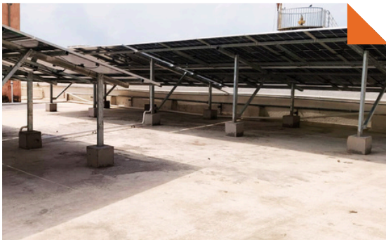
Shree Samdadi Bhavan (100 kWp)
