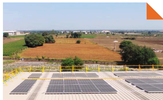
Max Power Engineers (49.5 kWp)
