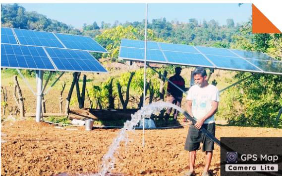
DGVCL (2760 Nos. Solar Water Pump)
