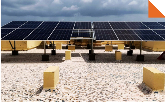
Shri Kolhapur Bhavan (49.5 kWp)
