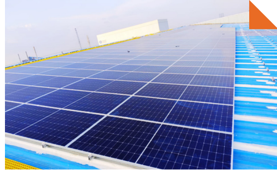
Ratnatris Pharmaceuticals (500 kWp)
