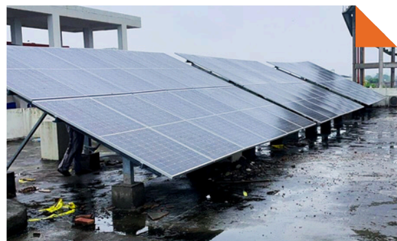
PEDA - Grid Tied Solar Plant (1470 kWp)
