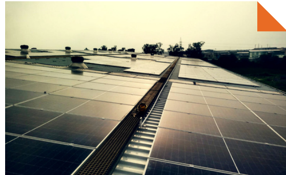
Embee Screens (378.36 kWp)
