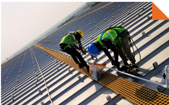
Topre India Pvt. Ltd. (1,173.70 kWp)
