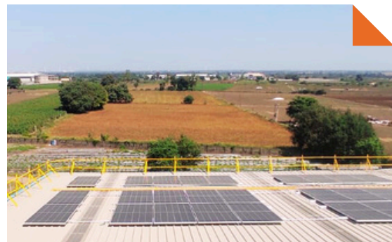
Max Power Engineers (49.5 kWp)
