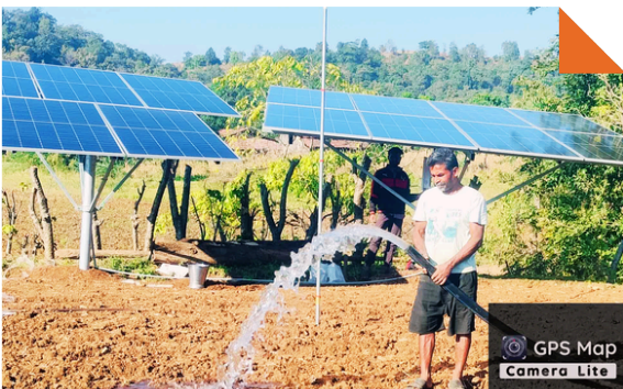
DGVCL (2760 Nos. Solar Water Pump)
