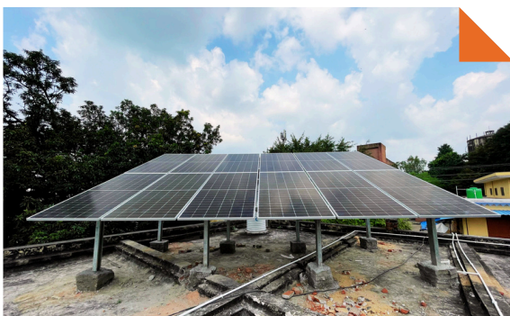
UPNEDA - Grid Tied Solar Plant (1400 kWp)
